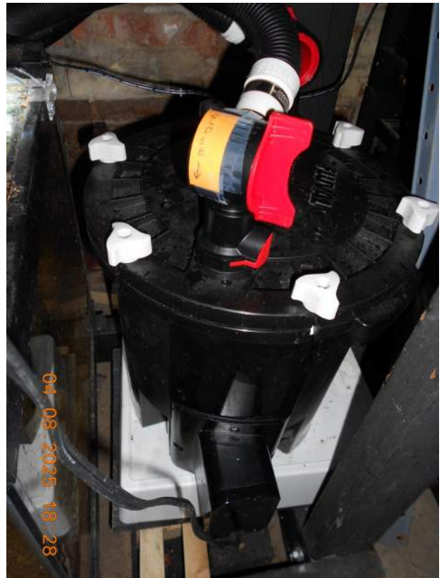
The FX2 is installed under its aquarium. Note the handwritten note taped to the output valve indicating which way to turn the red AquaStop valve. Not visible: the identical input valve.
